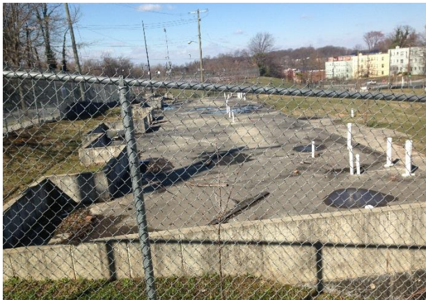
The Call Street slab: a monument to failure
